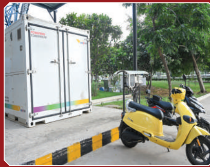
SMART HYBRID MICROGRID- BATTERY ENERGY STORAGE (100 KWH)
